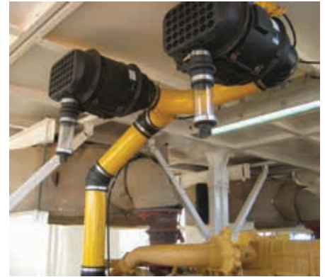
Dust Dumpa + PSD air cleaners extended the filter service life for a geothermal drill rig in Australia.
